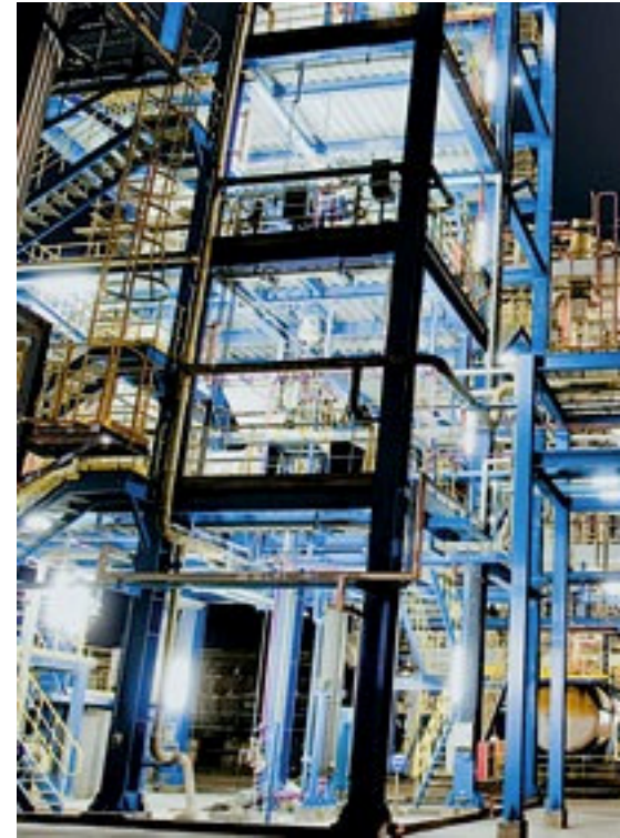
Arkema’s Changshu Haike facility in Jiangsu, China receives HFC-23 destruction credits through the CDM that effectively subsidize HCFC-22 production.
