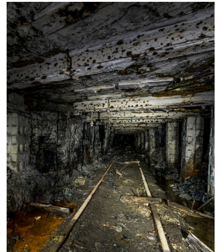
Above: Methane management policies are an essential part of mine closure plans.
