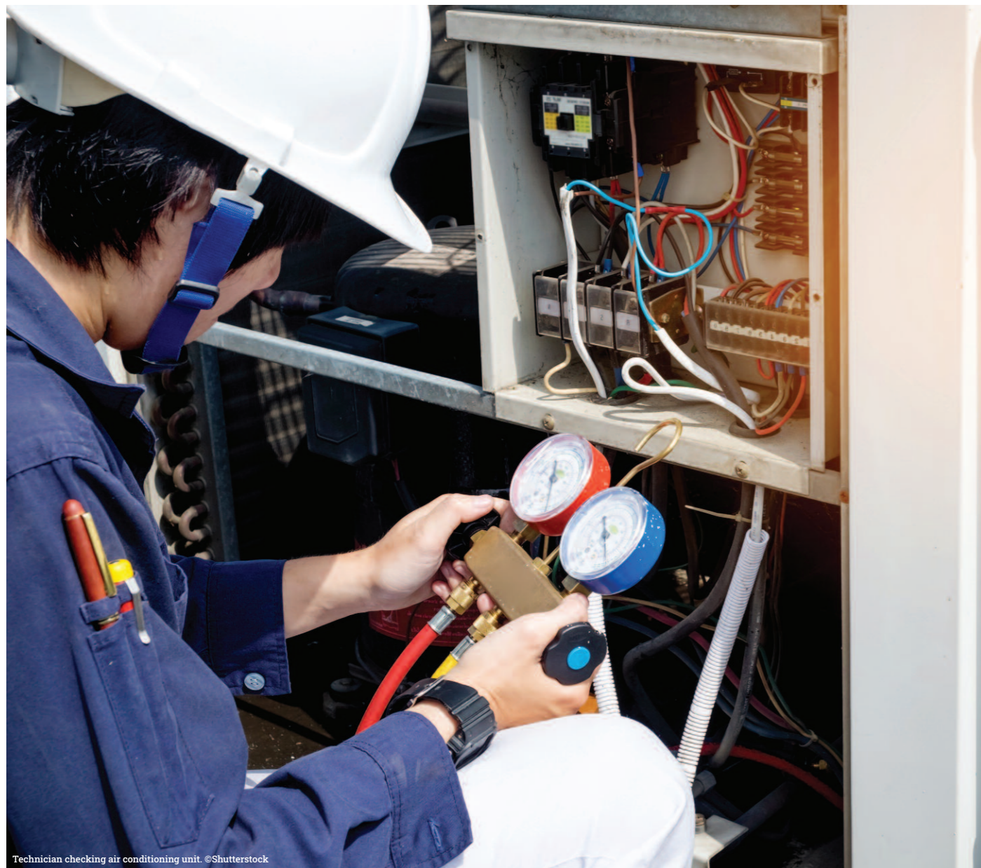
Technician checking air conditioning unit. ©Shutterstock
